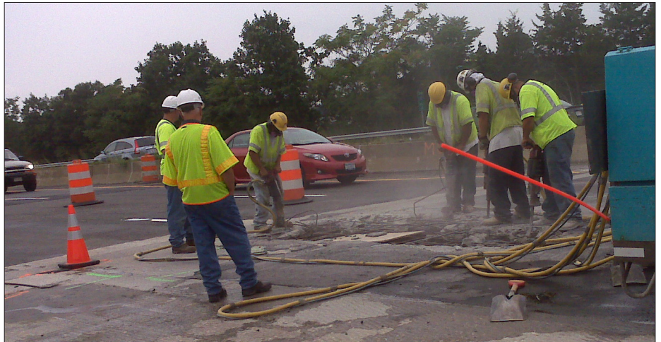
Cities and towns can save millions in road repairs by continuously evaluating pavement conditions.
